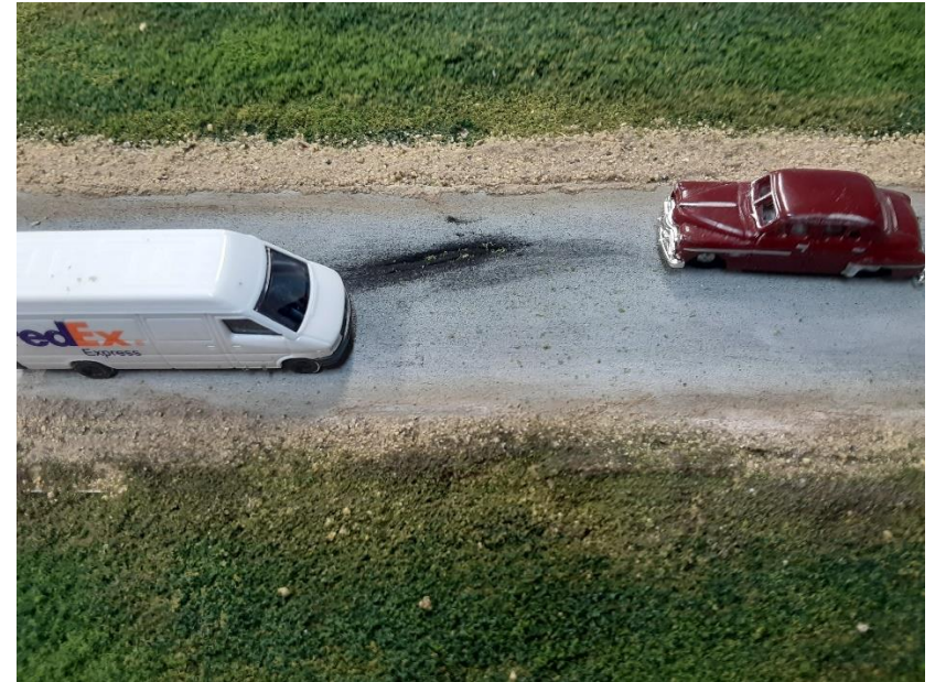
Soft black foam-asphalt with patched hole
